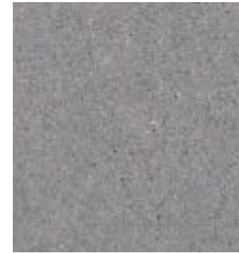
Concrete surface with no aggregate exposure.
